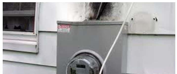
Service entrance destroyed by a surge
