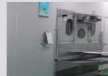
Automatic spray gold production workshop
