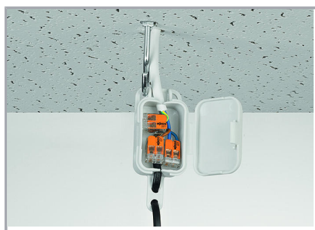
Pendant light connection in a suspended ceiling
